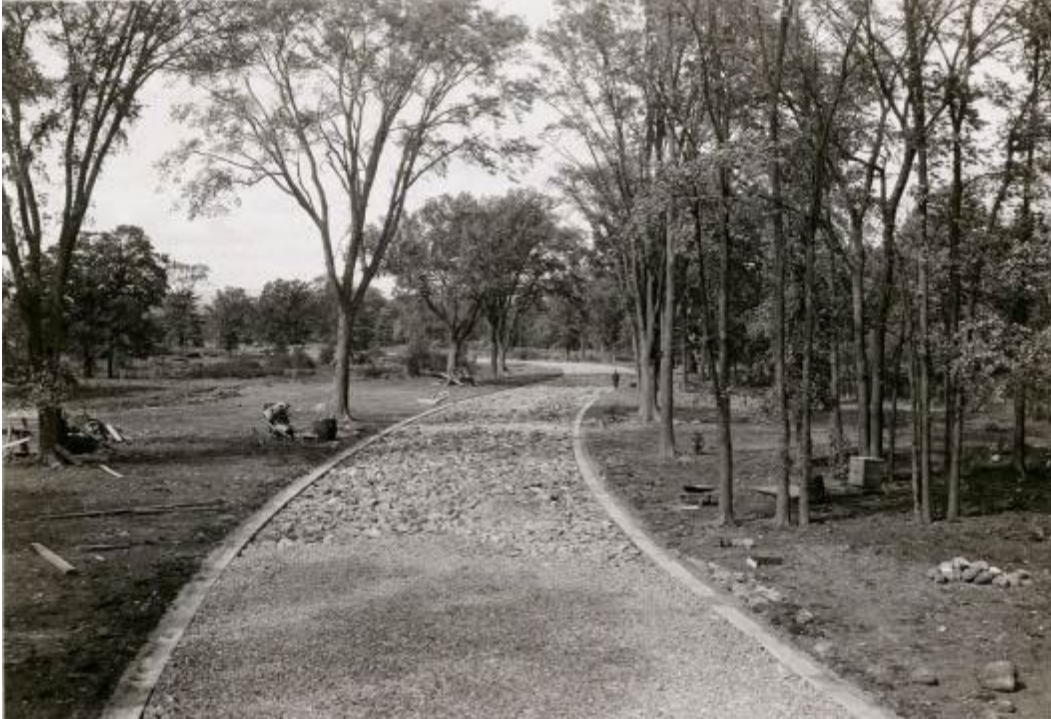
Figure 13: Image of macadamized construction phase 1 of West End Driveway facing south of Ottawa River, LAC
